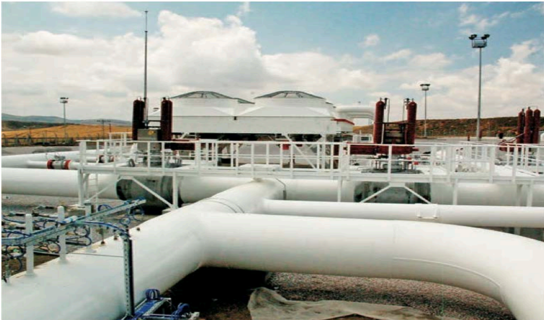
Figure 9. Compressor station (Source: BOTAS)
