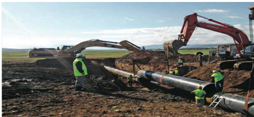
Figure 15. Transmission Line (Source: Botas)
